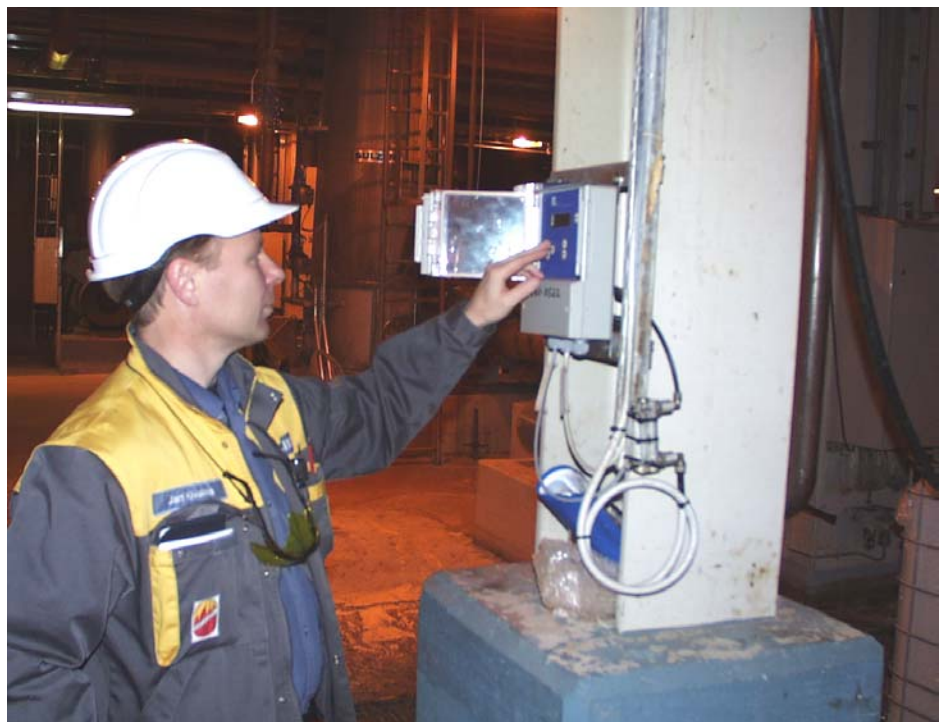
Mr. Jari Kivakka is in charge of the maintenance of automation in Kemi pulp mill.
